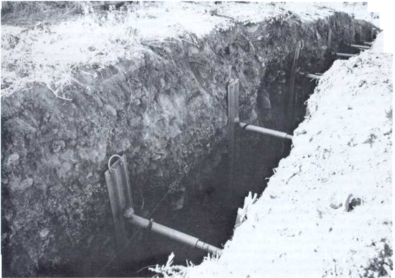
Figure 5-38.—Trench excavation showing hydraulic trench jack shoring. Trench 1, Pyramid Lake, Nevada (October 1983). P801-D-81042.
