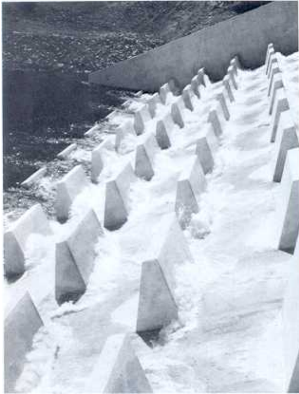
Figure 9-17.—Baffled chute drop spillway. Conconully Dam, Washington. The flow shown passing over the spillway is about 50 ft 3 /s. P21-141-178NA.
