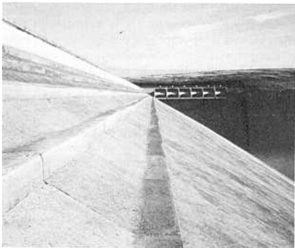
Figure 6-47.—Paved upstream slope of an earthfill dam. Dam is in excellent condition after 40 years of service. The structure is McKay Dam on a tributary of the Umatilla River in Oregon. 288-D-2878.
