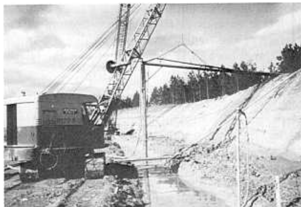
Figure 6-20.—Airlifting sand from bottom of slurry trench (U.S. Army Corps of Engineers). 288-D-2895.
