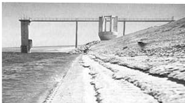
Figure 6-53.—Soil-cement paving on the upstream slope of Cheney Dam, Kansas. The soil-cement is in excellent condition after numerous storms. P835-526-1006NA.
