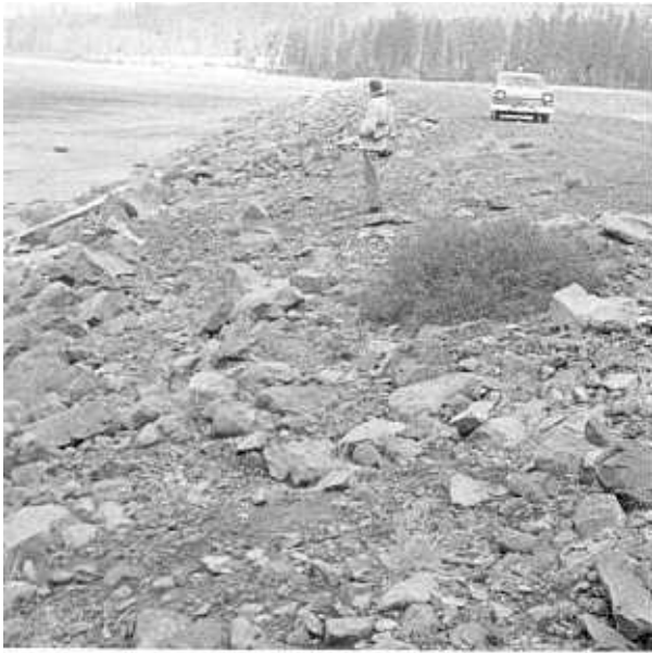
Figure 6-49.—Displacement of riprap on a low dike by wave action. 288-D-2936.
