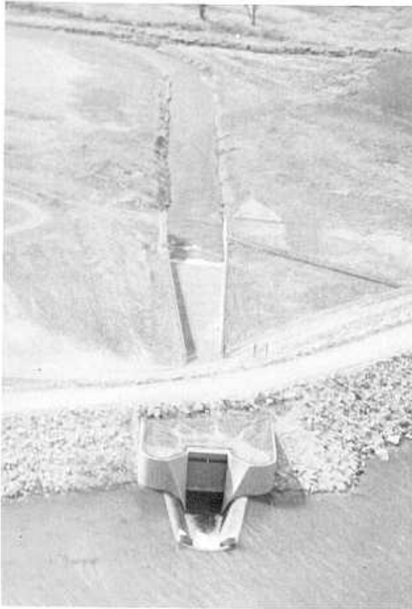
Figure 9-8.—Aerial view of service spillway. (Same spillway shown on figs. 9-7 and 9-9). 288-D-2896.
