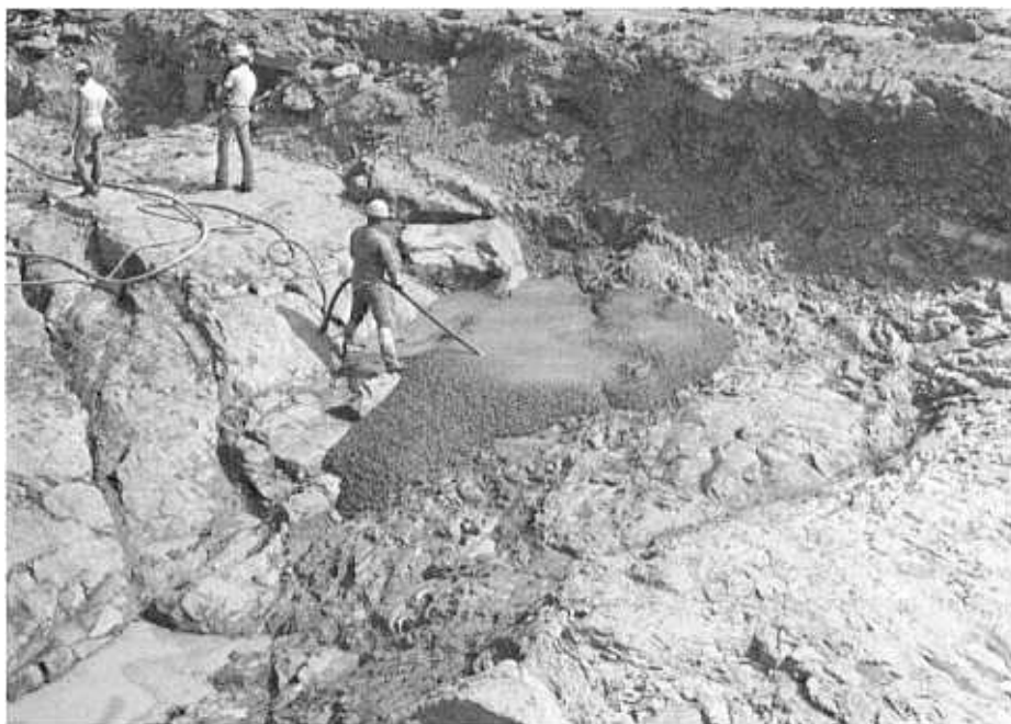
Figure E-3.—Cleanup of foundation rock. Dental concrete is used to fill an irregular surface in rock beneath the impervious zone. McGee Creek Dam, southeastern Oklahoma. P801-D-81035
