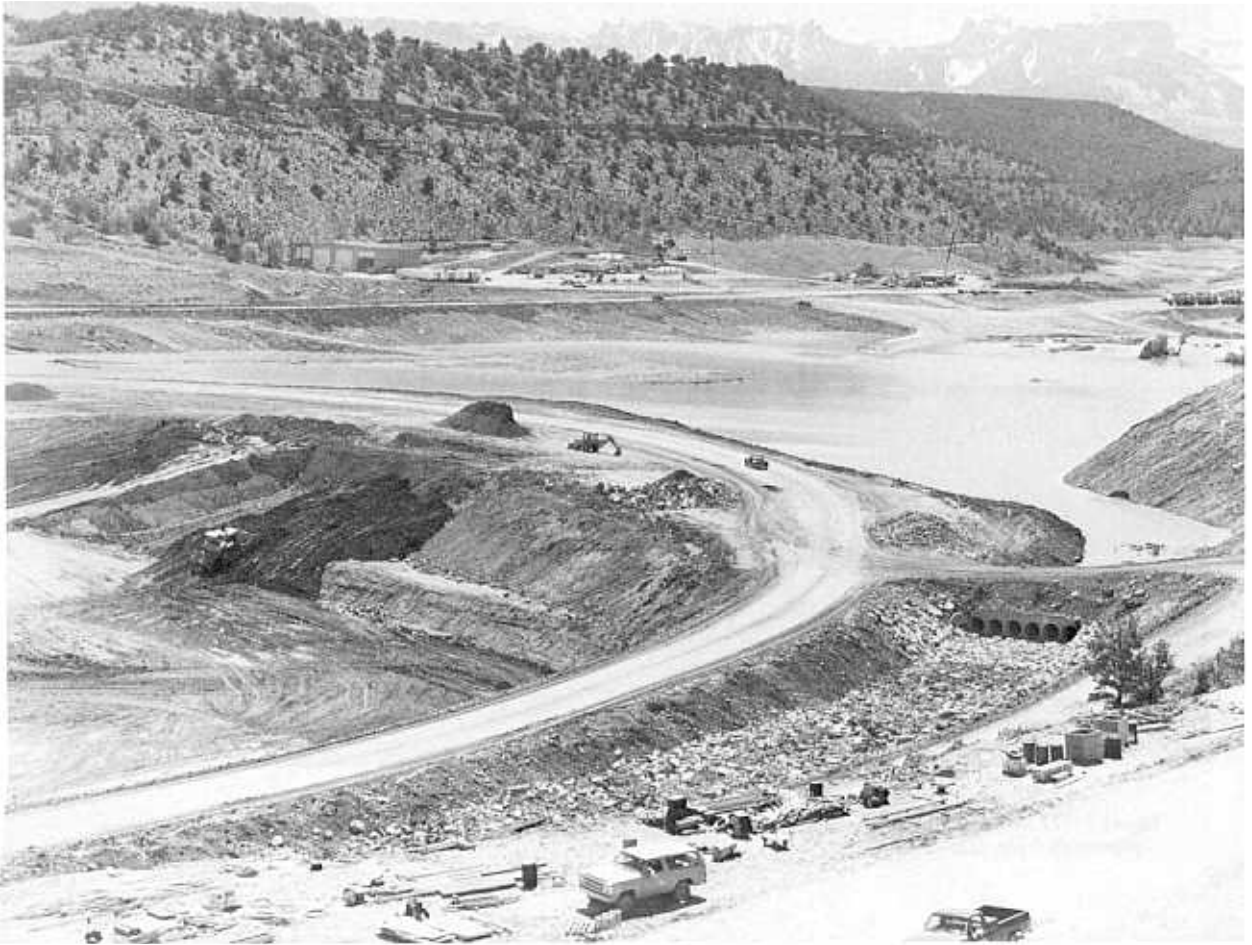
Figure 11-10.—Cofferdam at Ridgway Dam, Colorado. Note accumulation of water behind cofferdam and the temporary spillway that consists of six conduits on right side. P894-427-5989 NA.
