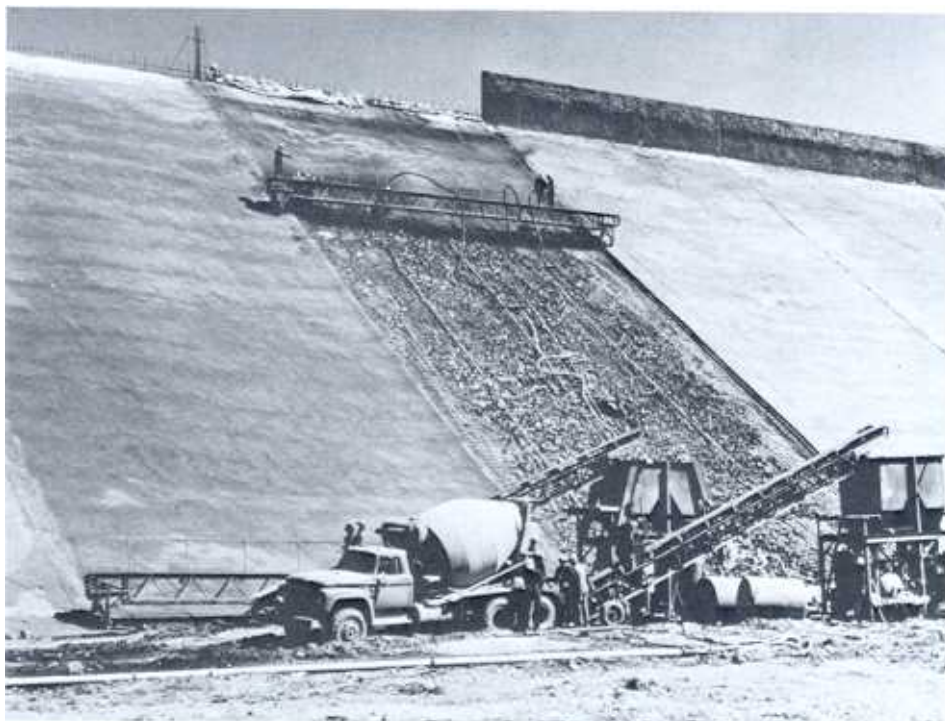
Figure 7-15.—Placement of shotcrete on the upstream face of Taum Sauk Dam, Missouri. (Union Electric Co. photograph). 288-D-2883.
