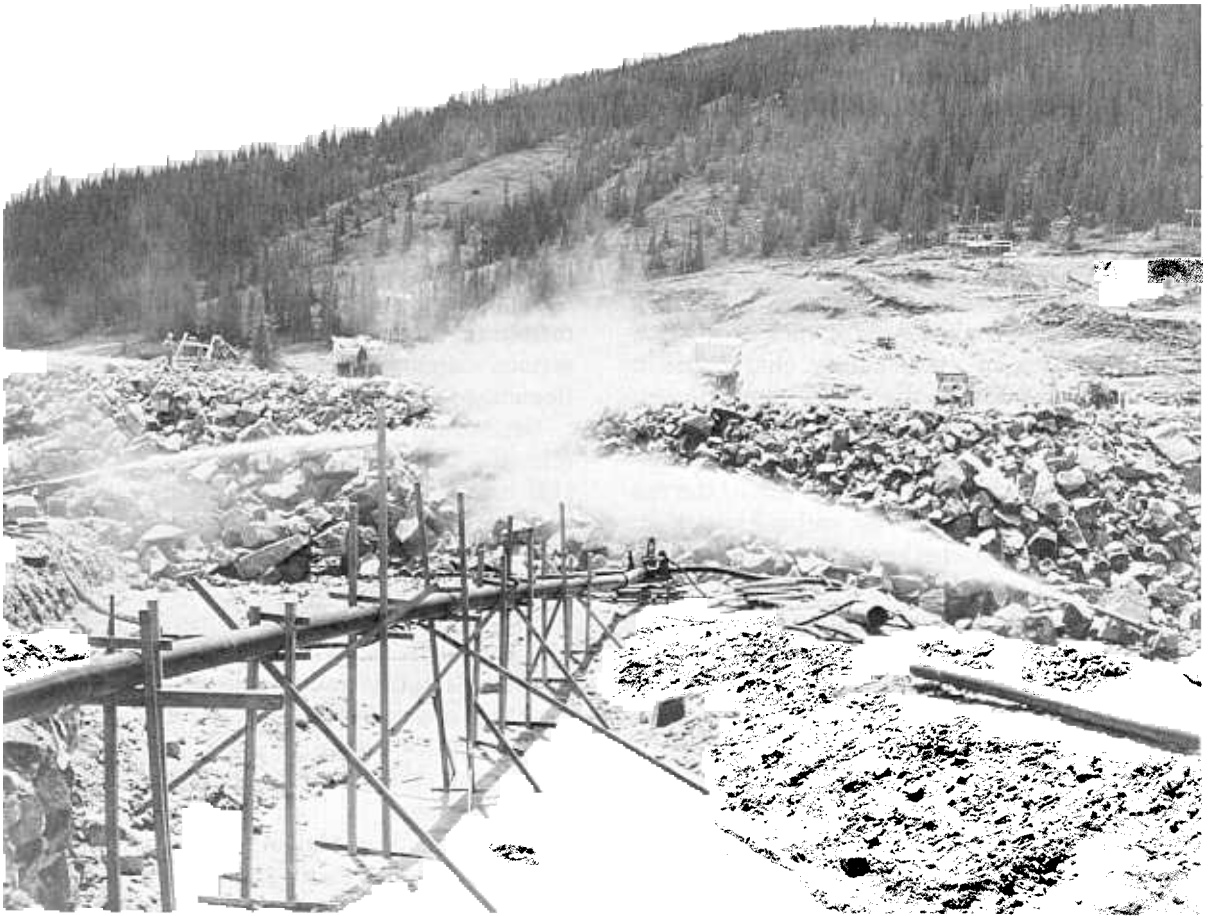
Figure 7-11.—Typical rockfill sluicing operation. Montgomery Dam, Colorado (Black and Veatch Engineers photograph). 288-D-2879.
