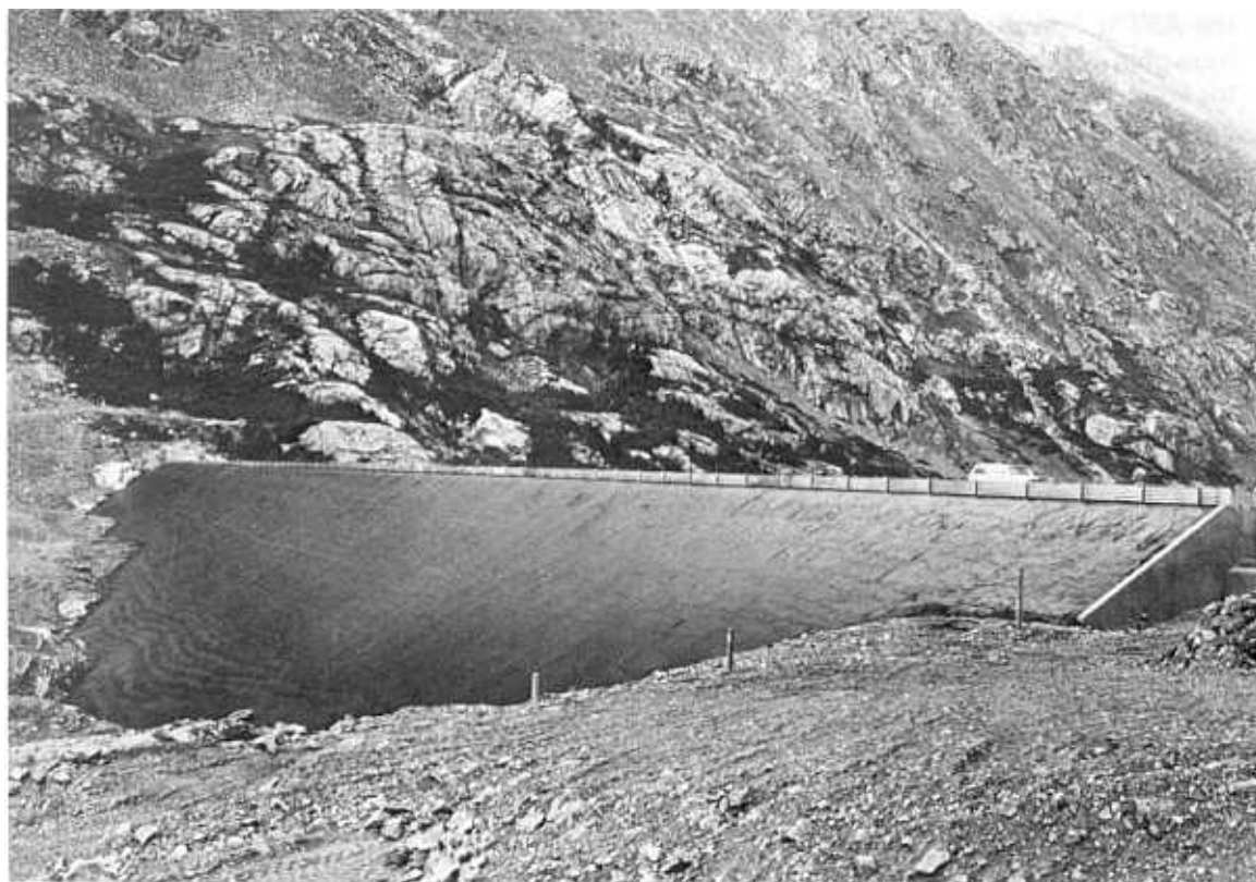
Figure 7-19.—Completed asphaltic-concrete facing at Upper Blue River Dam, Colorado. (Dept. of Public Utilities, Colorado Springs, Colorado, photograph). 288-D-2885.
