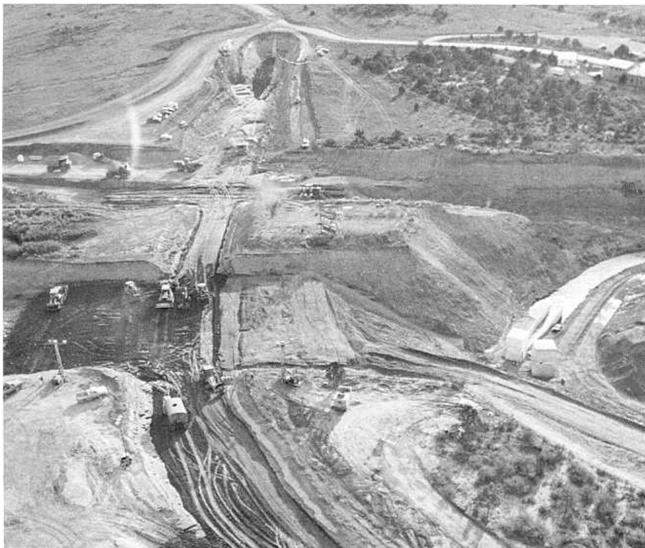
Figure 6-15.—Cutoff trench excavation and backfill. Great Cut Dike, Dolores Project, Colorado. CN71-438-10903NA.
