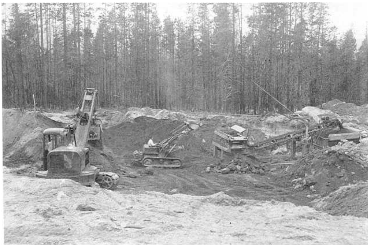
Figure E-8.—Removal of oversize rock by screening pit-run material. Impermeable borrow area for a small earthfill storage dam on Crescent Creek in Oregon. P806-126-55.
