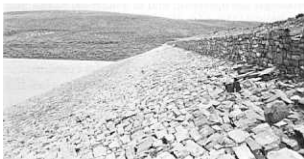
Figure 6.51.—Hand-placed rock riprap on Indian Creek Dike. An offstream dike for Strawberry Reservoir, part of a transmountain diversion project in Utah. 288-D-2935.
