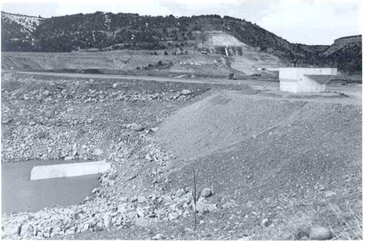
Figure 11-3.—Diversion through an auxiliary stream-level conduit. Intake structure (under construction) is at upper right. Ridgway Dam. P894-427-5891 NA.
