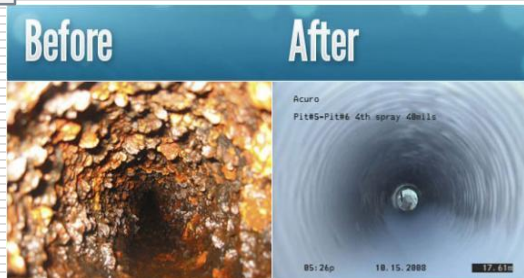
Pipe Tuberculation and Lining
